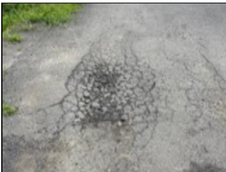
Figure 10 Differences in damaged photo locations by inspectors
