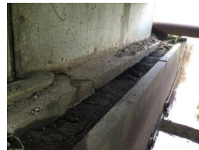
写真-1 点検調書判定III
