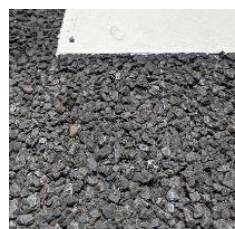
CWA 2 : Asphalt in the Big Sight parking lot is not suitable for racing asphalt. Aggregates are too loose. Re-asphalting of the Wearing Course necessary (e.g. 4 cm).
