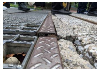
CWA 19 : Realignment and replacement of existing udrains with new ones. Concrete and asphalt renewal around the U-Drain. Replacement of U-Drain Cover with closed cover or temporarily close while maintaining drainage capacity.
