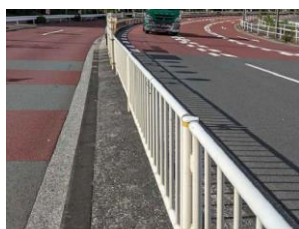
CWA 9 : Demolition of existing median island and vehicle restraint system. This area must be repaved.
