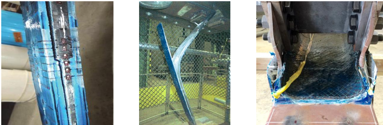
Fig. 1 Peeling failure on steel members bonding CFRP sheets.
