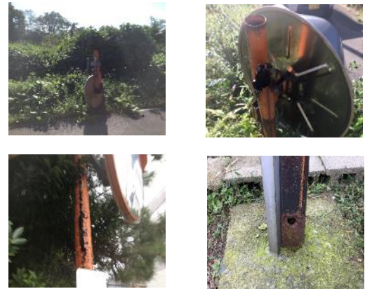
Fig.3 Photograph example of corrosion and break
